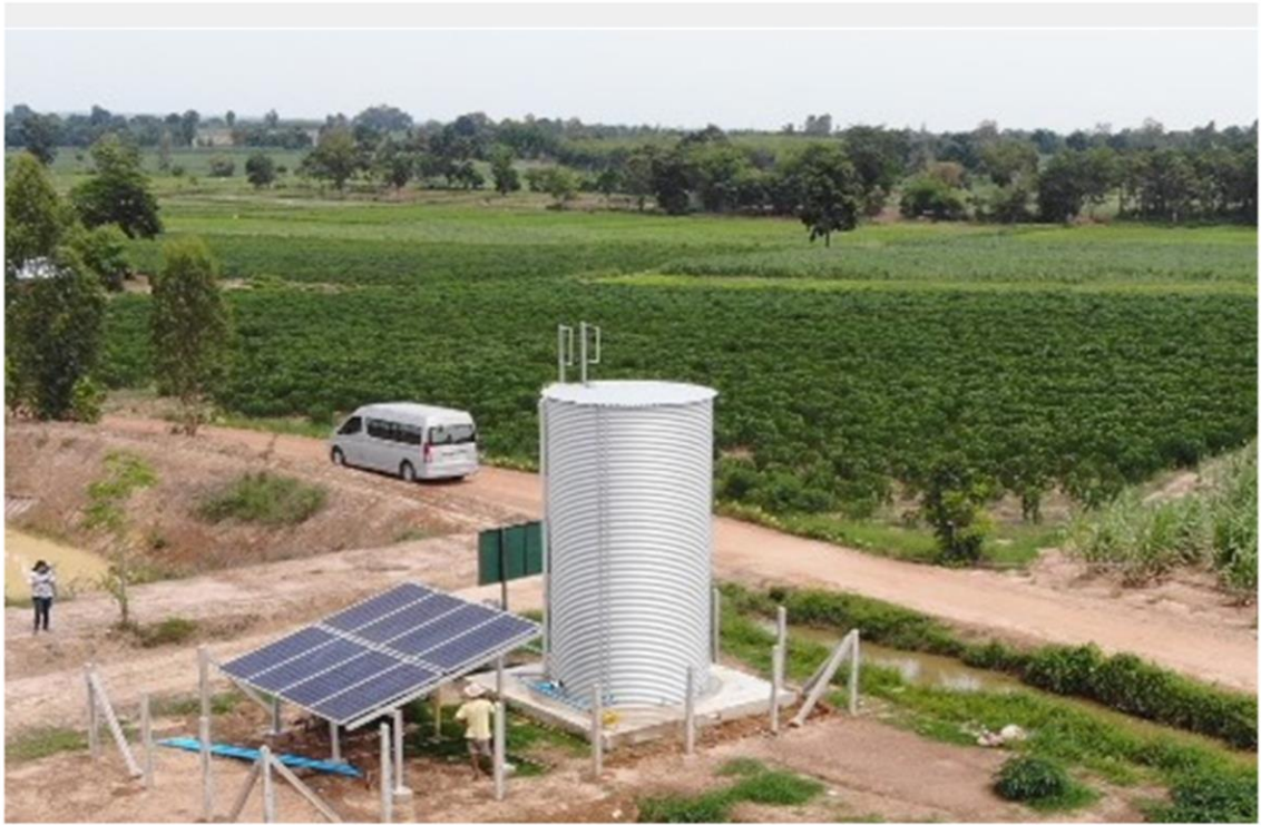
Water tank with solar cell RCT-15-57 (40,136 liters), Mahasarakham
