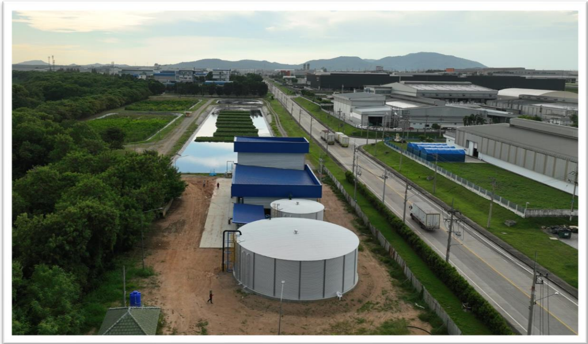
WHA-E1 RCT-470-50 (1,069,891 liters) Eastern Seaboard Pluak Daeng District, Rayong Province Diameter: 16.507 m H: 5 m For RO water and raw water storage in the water treatment centers installed on the industrial estate.
